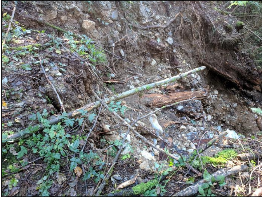
Photo 2: Slide scarp from the NSR above. The tension crack on the left side of the photo is about 10 cm wide.
