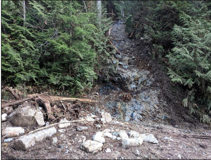
Photo 16: The landslide reached Lost Creek FSR where the road was constructed on bedrock. Note the bedrock exposed in the slide track.
