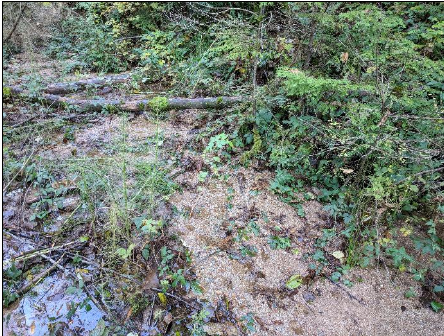
Photo 1: NSR above the scarp. The surface has standing water. Coarse sand has deposited on the road surface.
