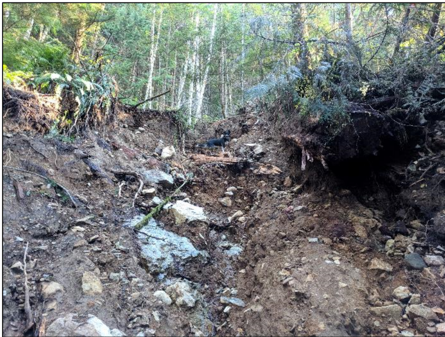
Photo 3: Looking at the scarp from below. The large log on the right side of the scarp is partially buried under the road surface above. The dog is near where the road fill was before failure.
