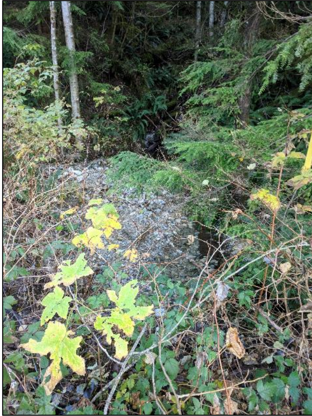
Photo 12: The CMP outlet at the bottom of the segment of the Lost Murdo FSR where the landslide sediment deposited. Some landslide sediment deposited in the forest at that outlet, but water is flowing through the culvert.
